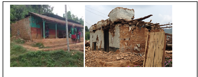
Figure 1: Photos of stone masonry buildings damaged by 2015 Earthquake in rural areas of Nepal.
